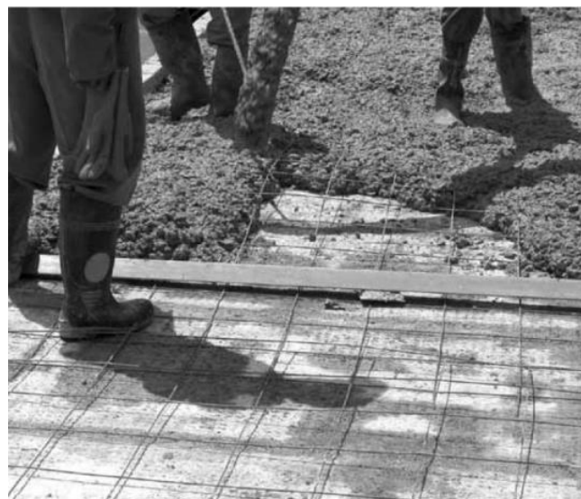
Pumping a concrete topping onto precast flooring. Reinforcement and screed battens in foreground.
