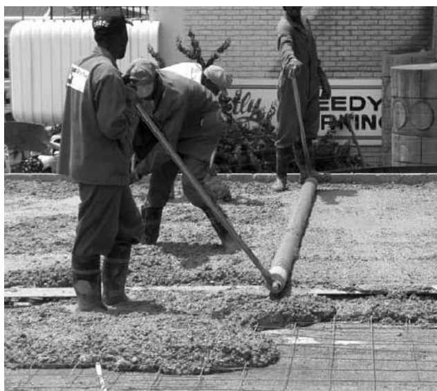
Levelling a concrete topping. Reinforcement and temporary screed battens in the foreground.
